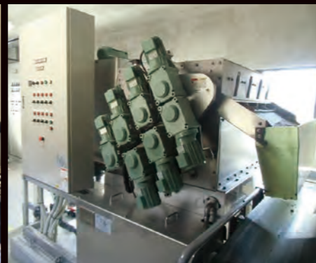
Excess Sludge at Noodle Production Plant (JD-1000)
